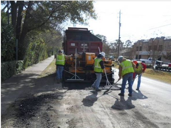
Placing Asphalt between Shady Glen and Carsey Lane north bound lane. View to the south.
