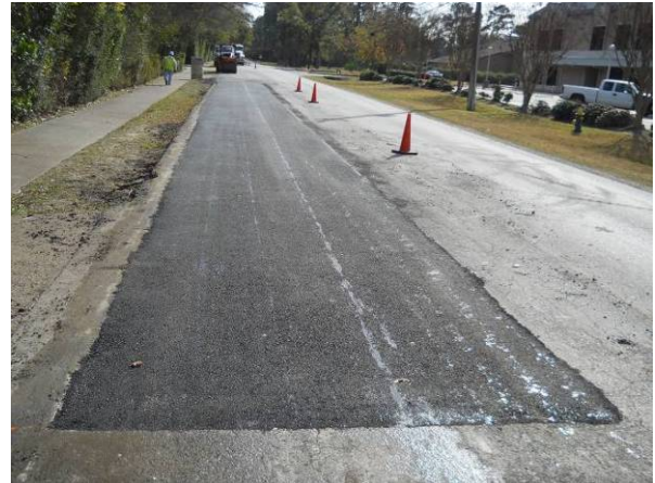
Road repair on the north bound lane between Jamestown and Shady Glen. View to the South.
