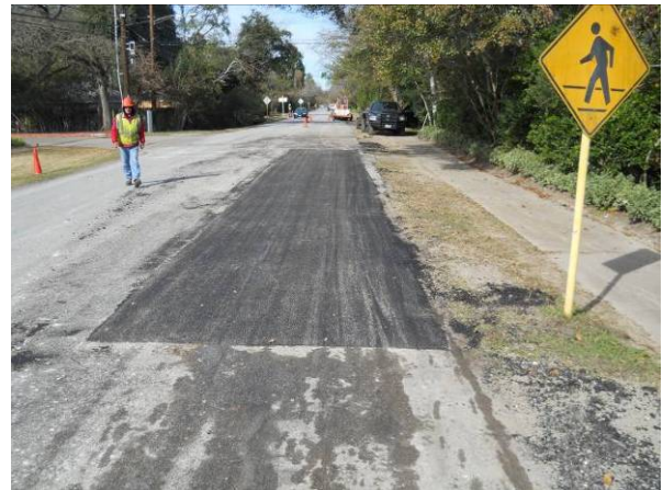
Road repair on the north bound lane between Shady Glen and Carsey Lane. View to the north.
