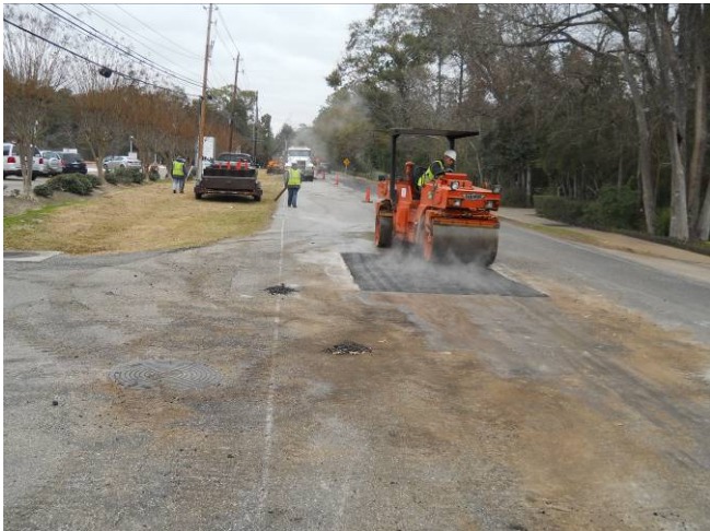
Rolling the asphalt repair in front of St Francis south bound lane. View to the north.
