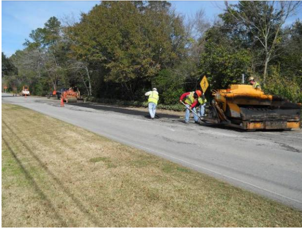
Placing the Asphalt on the N. bound lane in front of St. Francis. View to the northeast.
