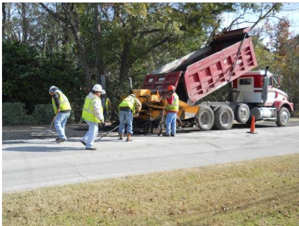
Placing the Asphalt on the N. bound lane in front of St. Francis. View to the southeast.
