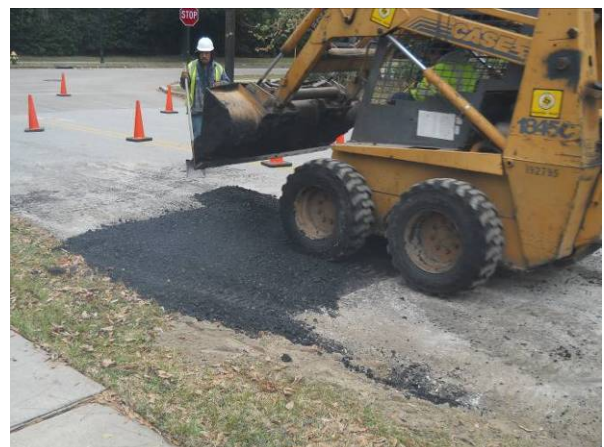
Placing the asphalt for the road repair on Taylorcrest @ Piney Point. View to the east.
