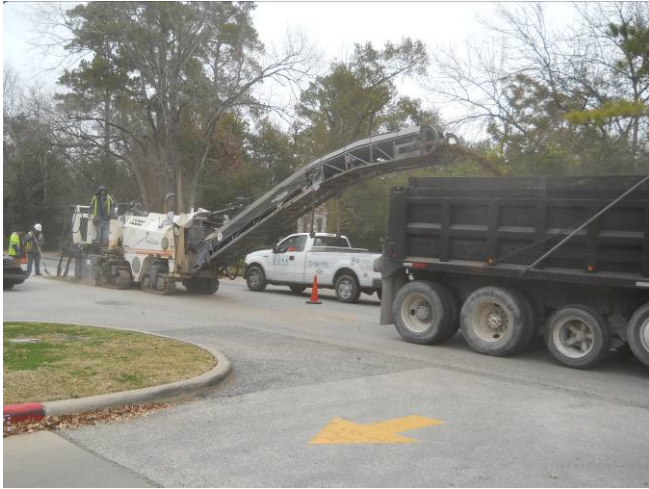
Chipping out the old asphalt in front of St Francis south bound lane. View to the north.
