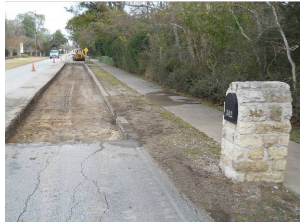
Asphalt repair on N. Piney Point between Shady Glen and Carsey Lane north bound lane. Removed the old Asphalt. View to the north.
