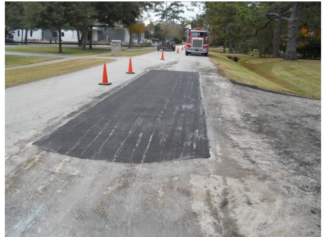
Asphalt repair at N. Piney Point and Chuckanut south bound lane is completed. View to the south.
