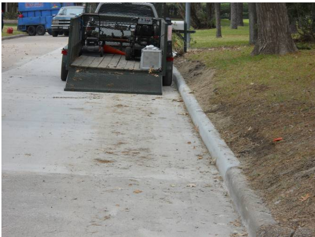
Cleaned up and backfill behind the 6-inch concrete curb at Meadowick Drive. View to the west.
