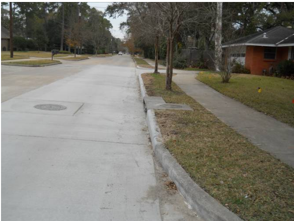
Cleaned up and backfill behind the 6-inch concrete curb place on Piney Point at Surry Oaks Lane. View to the north.
