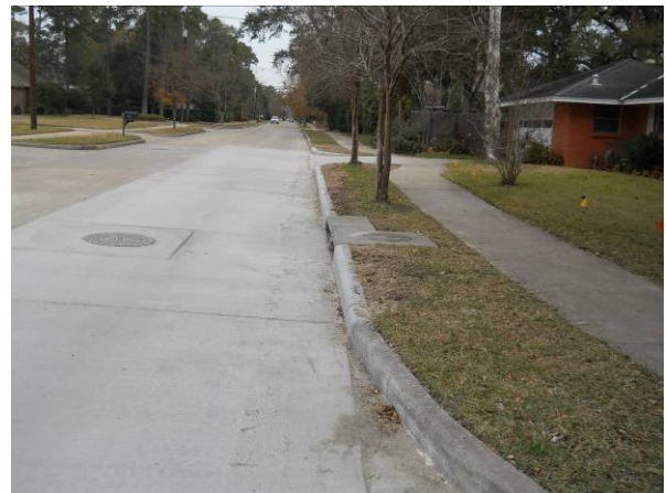
Placed concrete for the road repair at 11114 Meadowick Drive. View to the east
