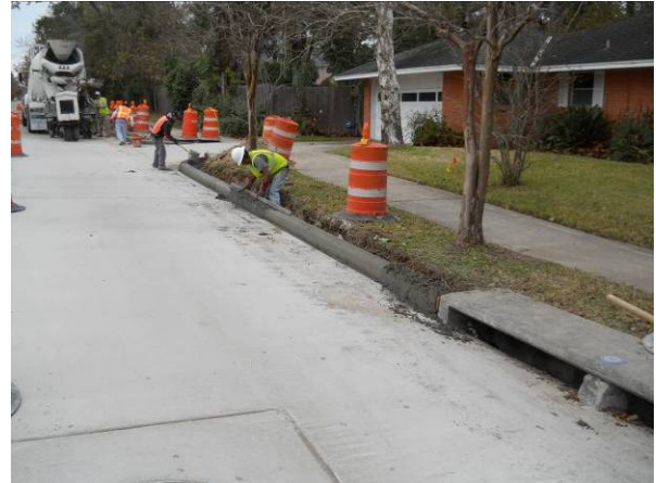
The 6-inch concrete curb is being placed on Piney Point at Surry Oaks Lane. View to the northeast.
