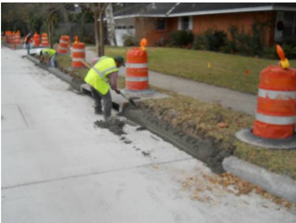
The 6-inch concrete curb is being placed on Piney Point at Surry Oaks Lane. View to the northeast.
