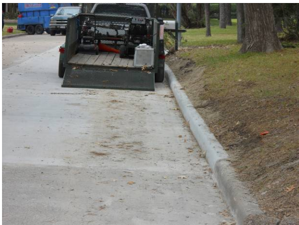
Placed the 6-inch concrete curb on Meadowick Lane road repair. View to the north.
