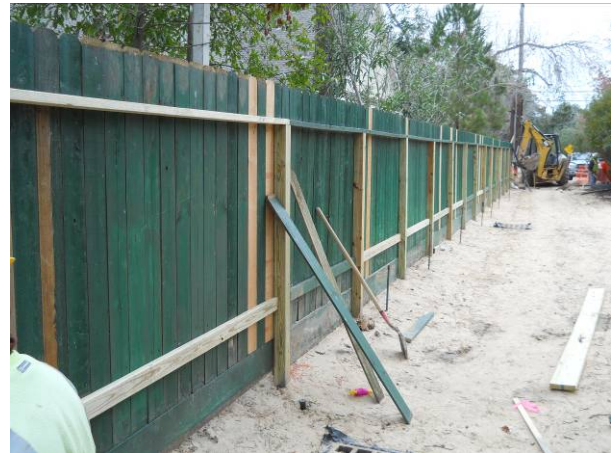
Contractor installed the wooden fence between Piney Point and Gingham at 439 Piney Point. View to the east.
