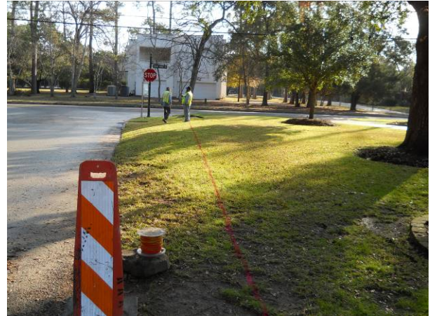
Contractor marked out the location of the new storm sewer line location on Calico Lane and Piney Point road.
