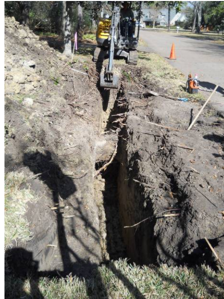
Excavating for the water line off set on Tynebridge Lane View to the north.
