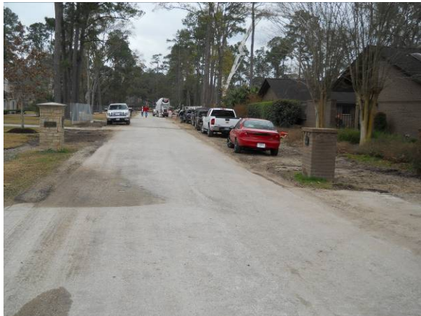
Contractor had dressed up the sides of Jan Kelly. Home contractors worker parked on the dress up area of Jan Kelly leaving ruts. View to the south
