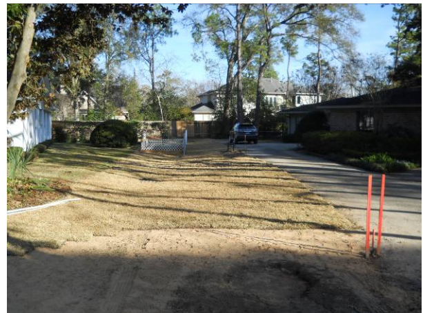
The contractor placed more sod grass in the easement between 426 and 430 Gingham Dr. View to the east.
