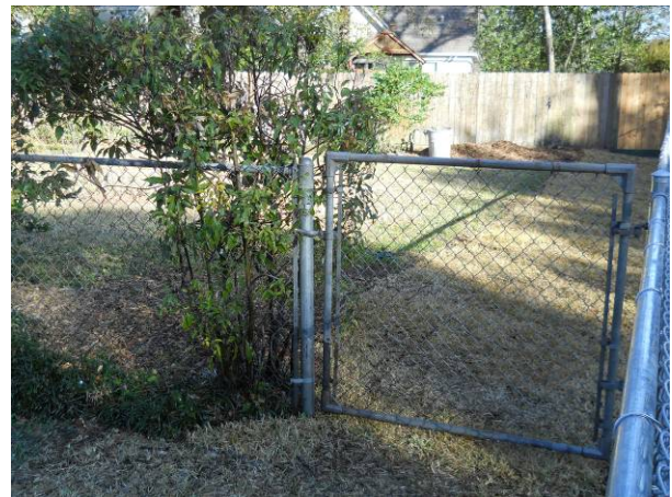
Contractor placed the sod grass and repaired the gate at 430 Gingham Dr, View to the east.
