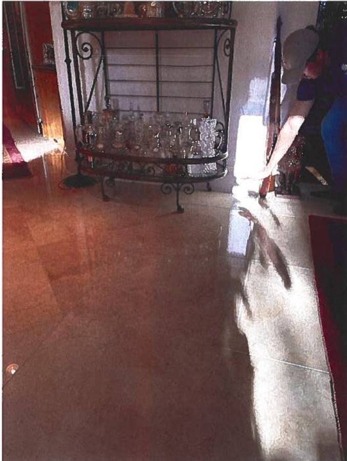
Where water levels got into house during Harvey.
